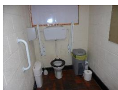
Grab bar fittings not compliant and poor contrast to walls
