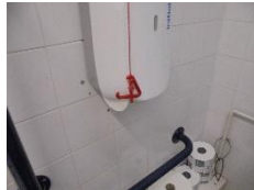
Alarm cord too short
